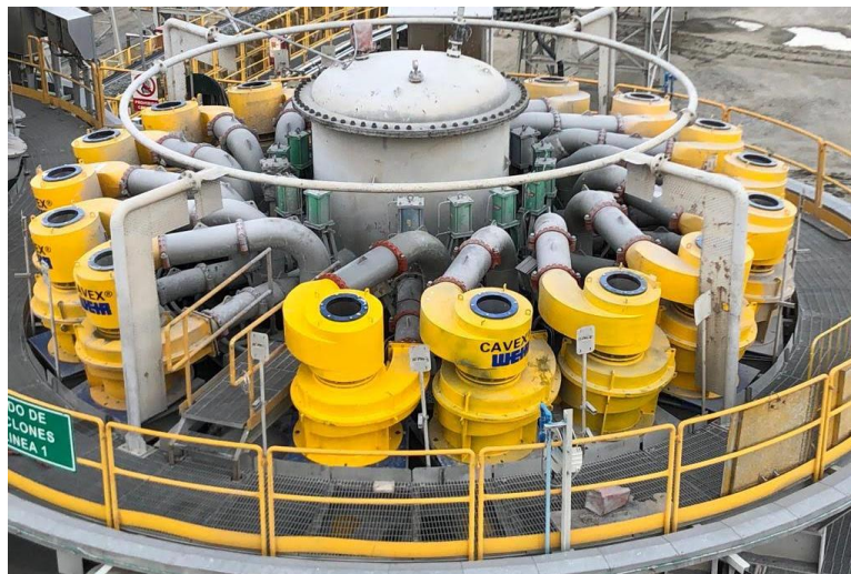
Figure 5—Photos of Cyclones Cavex with ACB Devices Installed at Constancia Grinding Circuit
