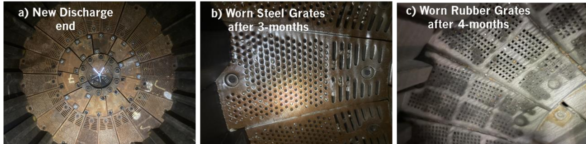
Figure 11: a) Mill#2 with grate-EEPL discharge end and b) worn steel grates after 3 months c) worn rubber grates after 4 months.
