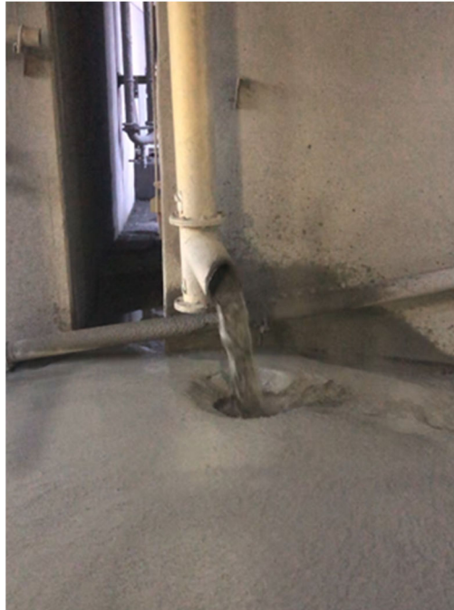
Figure 13—Ball Mill Trommel Oversize Chute Discharge to Drive Through Sump
